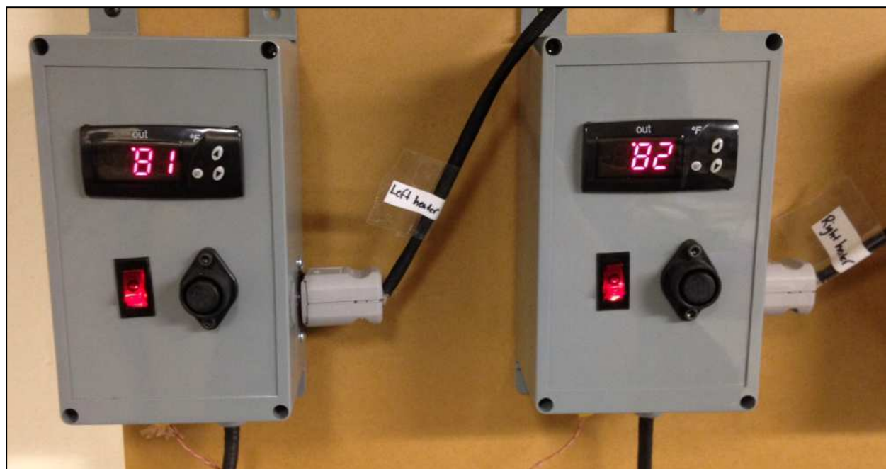
Figure 7: DP -7000 Controllers for Heaters
